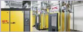
Air Compressor Heat Recovery
